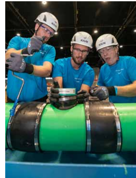
From left, Malte Olsen, Magnus Hansen, and Frank Davidsen of the Aarhus Vand Great Danes install an Inserta Tee® into a stretch of PVC pipe during the Collection Systems Event. Kieffer Photography
