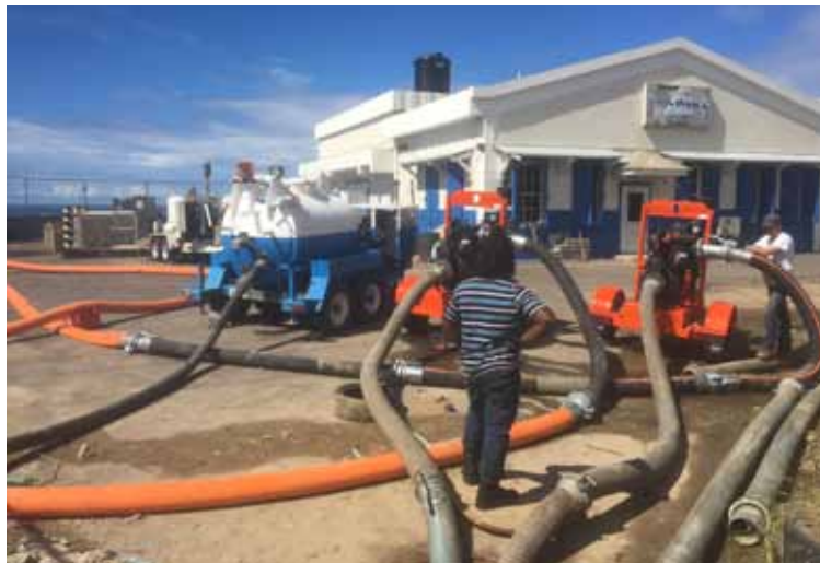
A maze of pumps needed to be set up to begin restoration work in Dominica. Marcel Misuraca, Ontario Clean Water Agency
