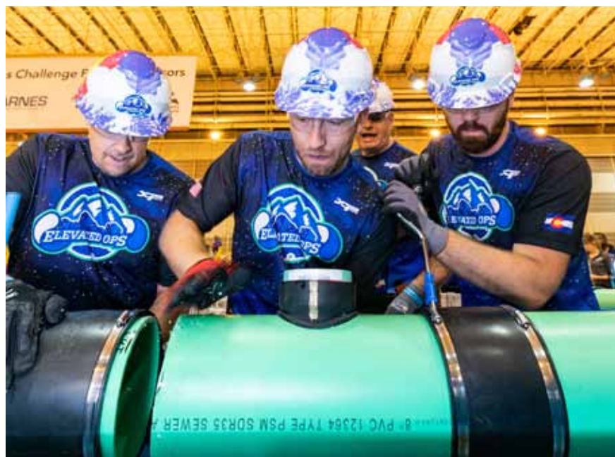
Lance Wenholz, Matt Duncan, Kelsey Gedge, and Josh Malloreoy pitch in to complete a pipe repair in the Collection Systems Event. Kieffer Photography
