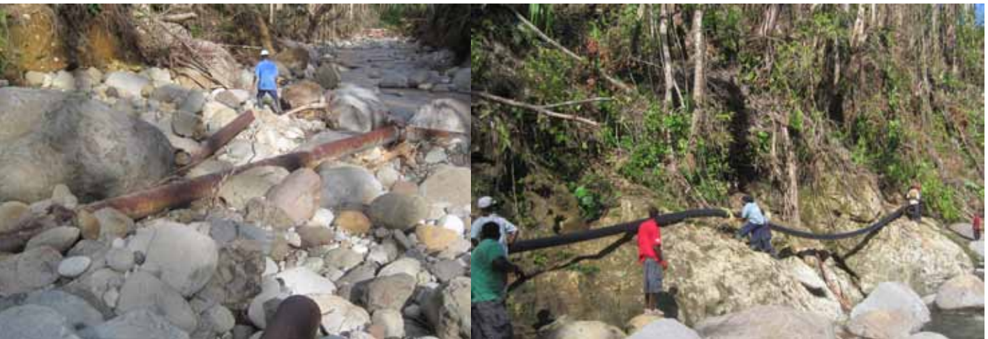
Left, an old water distribution pipe damaged during Hurricane Maria lies on a river bed in Dominica. Right, a new distribution pipe is being hung along the river. Marcel Misuraca/Ontario Clean Water Agency
